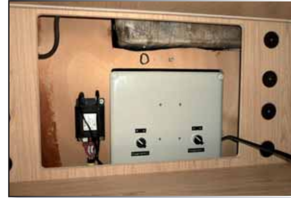
OVERRIDE SWITCHES N° 6-7 - STARBOARD CABIN
