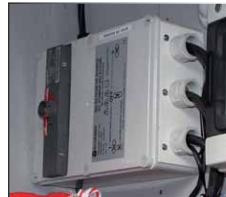
MANUAL SUPPLY SELECTOR SWITCH AIR CONDITIONING
