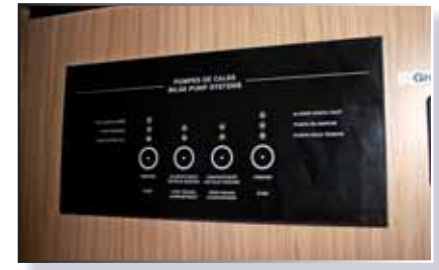
ELECTRIC BILGE PUMP SWITCHES
