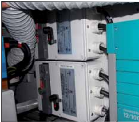
FORWARD SERVICE ROOM
