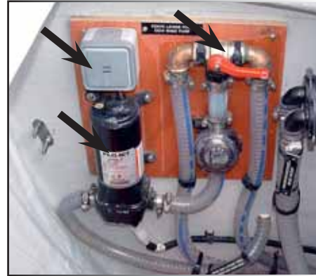
1 - 2 - POWER SWITCH + DECKWASH PUMP + SELECTION VALVE
