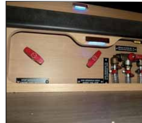
SHUT-OFF HANDLES FOR FUEL VALVES TO STARBOARD
