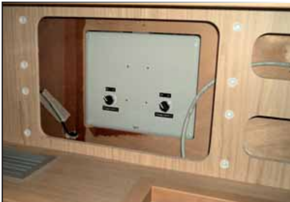
OVERRIDE SWITCHES N° 2-3 - PORT CABIN
