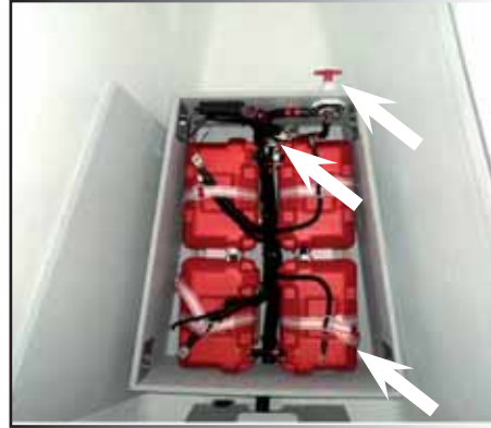
1 - BATTERIES + FUSE + CUT-OUT
