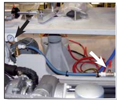
8 + PRESSURE GAUGE + WATER CIRCUIT REPRESSURIZATION VALVE
