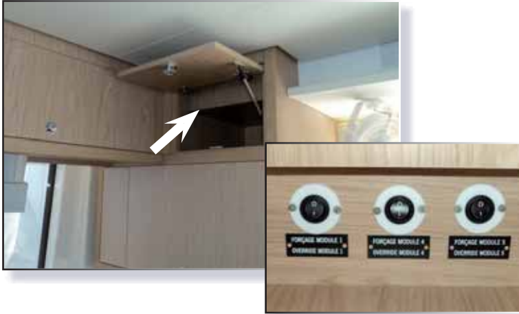
OVERRIDE SWITCHES N° 1-4-5 - GALLEY
