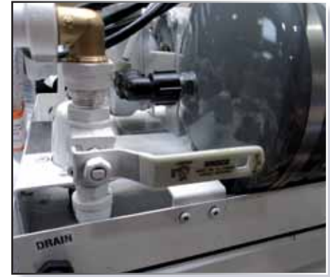
WATER ADDITION VALVE CONTROL
