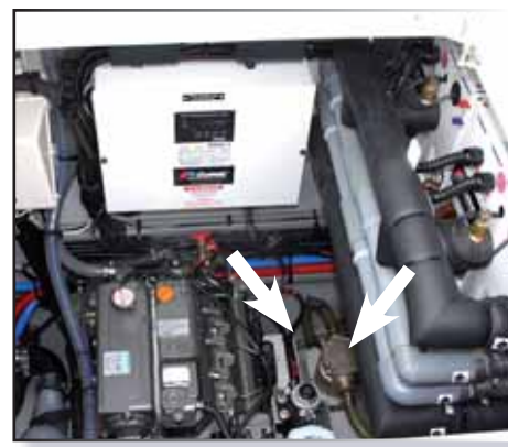
6 - AIR CONDITIONING UNIT SEA WATER INLET VALVE + FILTER
