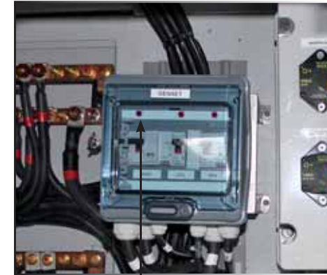
6 - AUTOMATIC BREAKERS OF THE GENERATOR
