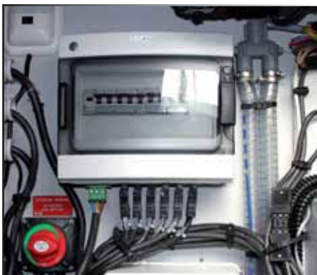
AIR CONDITIONING UNIT AUTOMATIC BREAKERS
