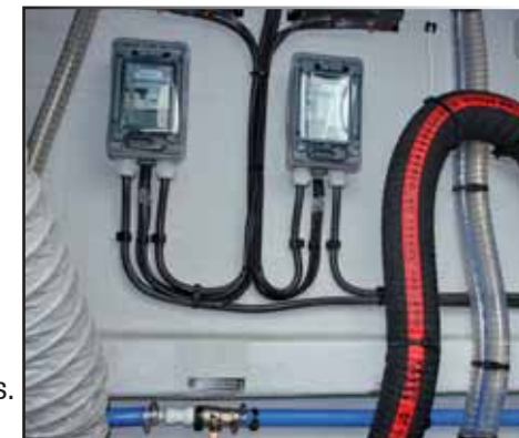
13 - AUTOMATIC BREAKERS OF THE SHORE POWER SOCKETS
