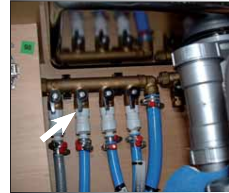
5 - DISHWASHER FRESH WATER SUPPLY VALVE
