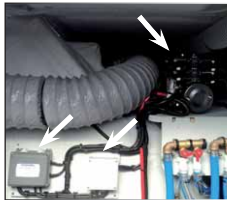
2 - HYDRAULIC PUMP + POWER SUPPLY BOXES
