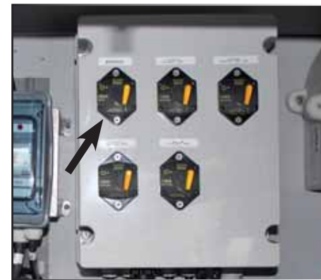
3 - AUTOMATIC BREAKER OF THE WINDLASS
