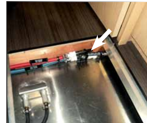
3 - WASHER DRYER FRESH WATER SUPPLY VALVE
