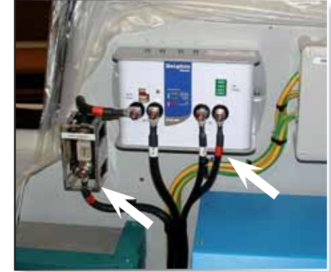
3 - BATTERY CHARGER + CHARGER FUSE
