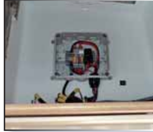
5 - ELECTRONIC FUSES BOX
