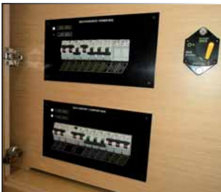
AUTOMATIC BREAKERS 110 V - 220 V + WATER PUMP
