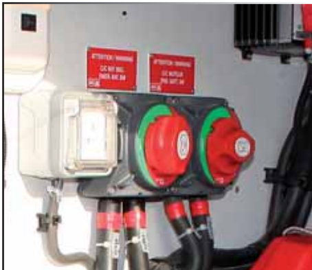
COUPLING + STARBOARD ENGINE CUT OUTS
