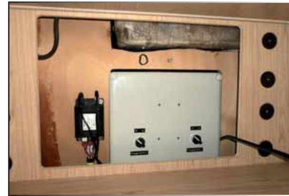
3 - OVERRIDE-SCHALTER Nr. 6-7 - STEUERBORDKABINE
